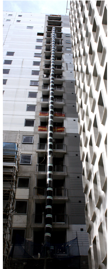
Mounted on Slab
