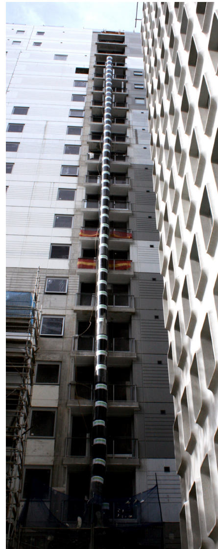
Mounted on Slab
